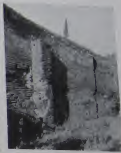
FIG. 183. SOUTHWEST PERIMETER WALL OF THE CHAPEL OF SAINTS STEPHEN AND PAUL. THE WALL WHICH SEALS THE SOUTH DOORWAY.
